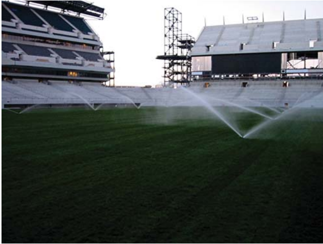
2. Underground, automatic irrigation system
